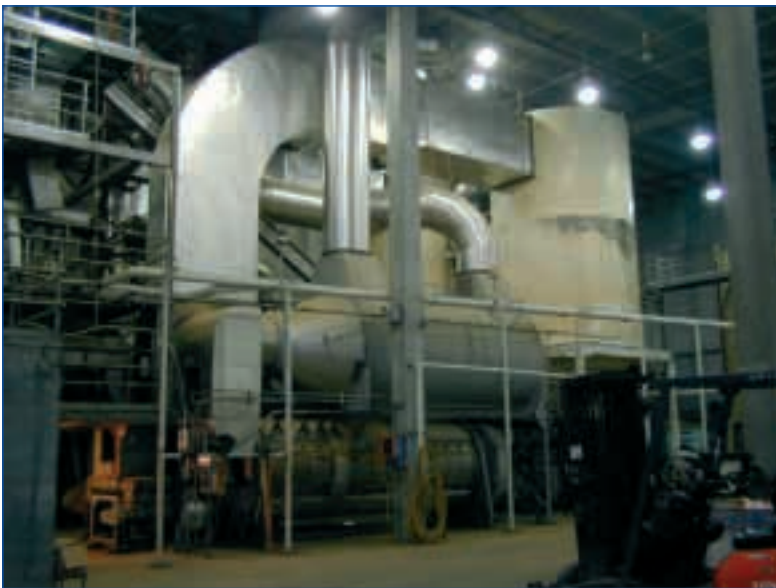
Large sludge drying plant
